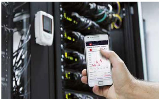
Control of climatic data from a data centre using the smartphone application
