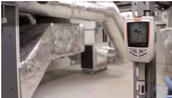
Magnetised KH 220 in the air conditioning room of an industrial facility
