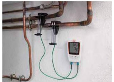
KTT 220 equipped with two clipped thermocouple sensors to control the domestic hot water network (DHW), mounted onto a wall plate
